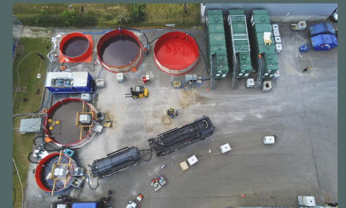
The separating system for the pumped oil and water mixture needs a lot of space – and found it on the ground of STAUB & Co. SILBERMANN in Gablingen.
